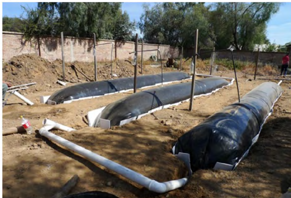
Fig. 1. The three tubular digesters in series, monitored in the Cochabamba slaughterhouse, at 2572 m above sea level ( Martí-Herrero et al., 2016 ).
